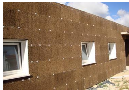
Figure 6. External insulation made of cork
