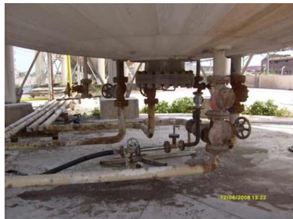
b) pipelines for streaming and filling
