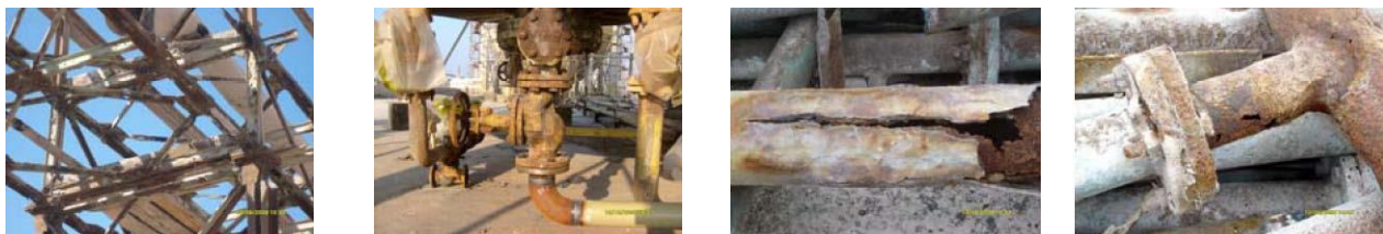
Figure 2. Examples of corrosion damage to pipeline steel structures [1, 2]
